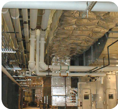
After installation, Grunau personnel balanced and commissioned the HVAC systems, including the air handling units, exhaust fans and more than 500 VAV boxes.
