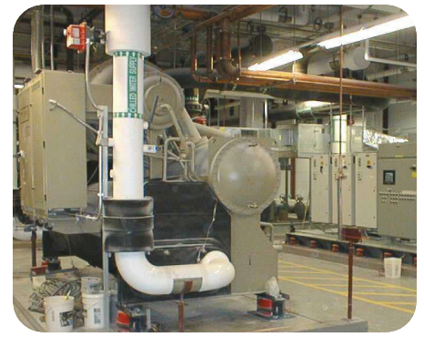
Grunau installed two 750-ton chillers in the penthouse level of the addition.
