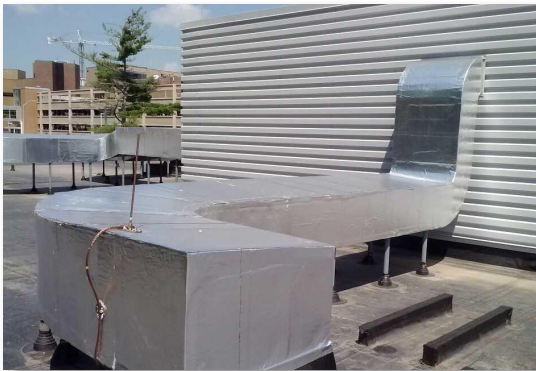
New HVAC ductwork leading into mechanical penthouse
